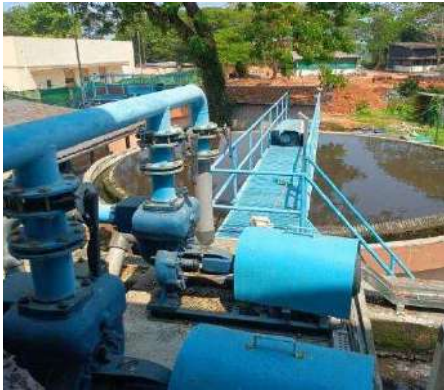
500 KLD STP at Kozhikode medical College
