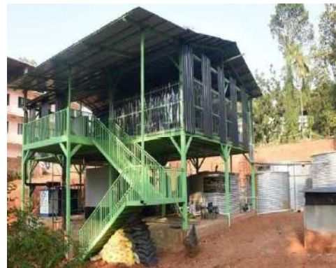
1 MLD STP at Kozhikode medical College
